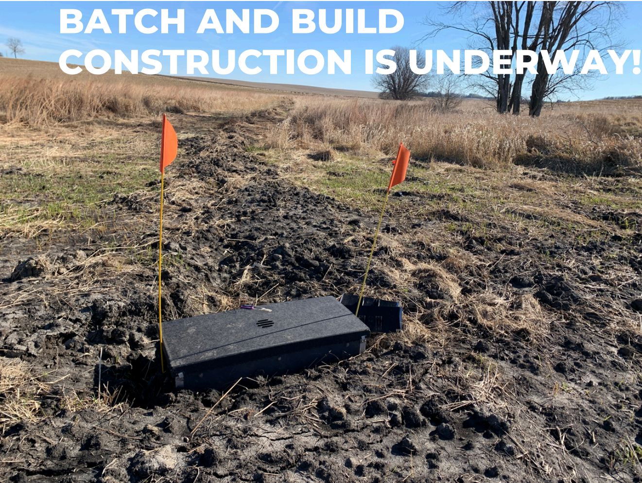
Above: Newly installed saturated buffer is already removing nitrates from tile water in a filter strip near West Branch.
